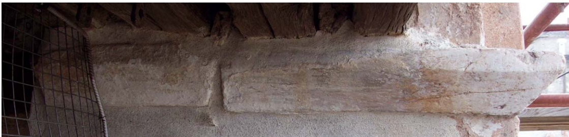
12 Vatopedi monastery; bell-tower; western wall-opening; undecorated cornices impacted in the southern arch
