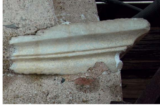
9 Vatopedi monastery; bell-tower; northern wall-opening; part of a door frame impacted in the eastern arch
