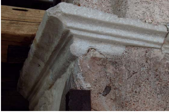
8 Vatopedi monastery; bell-tower; northern wall-opening; part of a door frame impacted in the western arch
