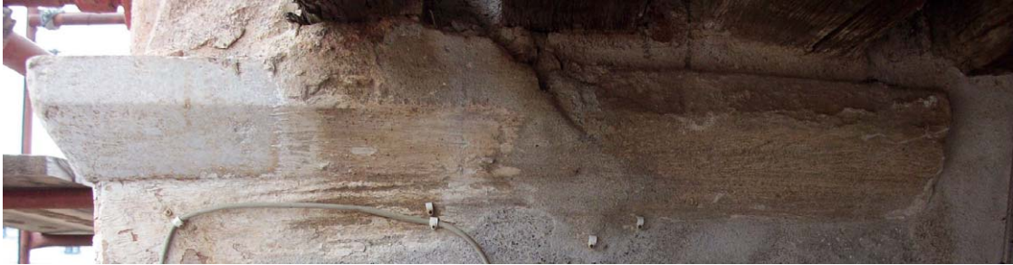
13 Vatopedi monastery; bell-tower; southern wall-opening; undecorated cornice impacted in the eastern arch
